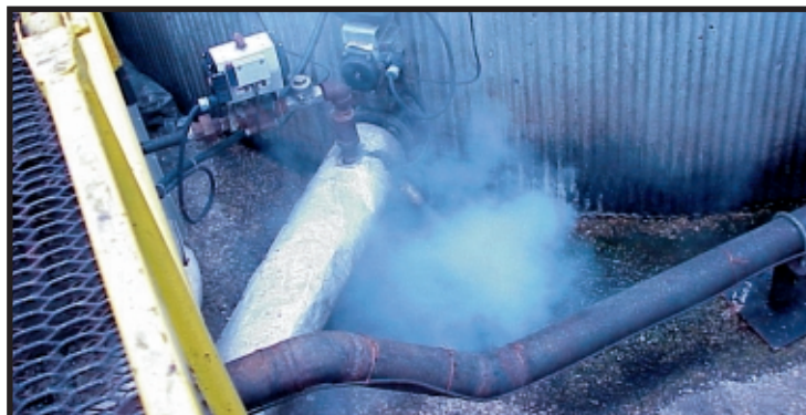
Correcting steam losses like this one has been a major factor in Unilever's impressive natural gas savings.
